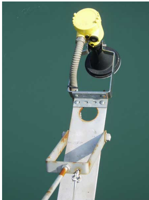
Figure 5. Level measurement by emerged radar. [© EDF DTG]
