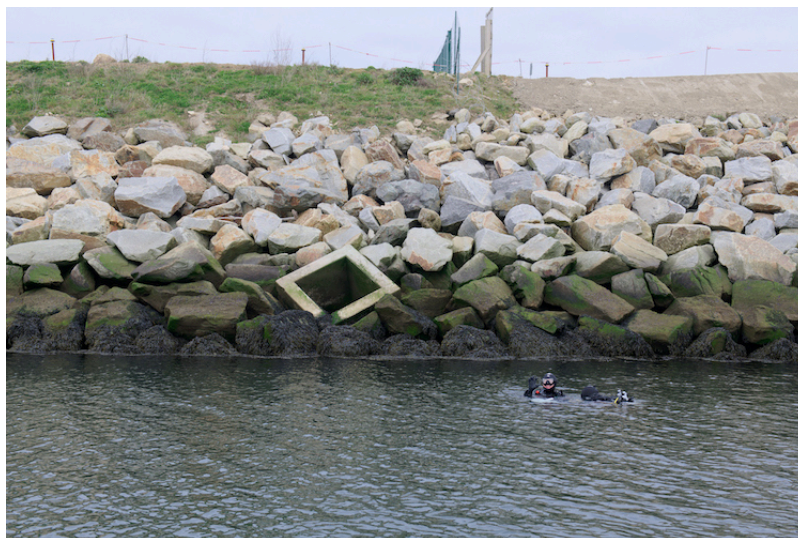
Figure 4. Example of an eco-block installed in the dike of the port of Brest (Bretagne-France). These eco-blocks remain filled with water at low tide, artificially recreating puddles characteristic of the rocky coasts of tidal seas. [Source © Ifremer - O. Dugornay]
