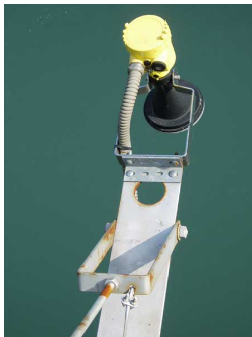
Figure 5. Level measurement by emerged radar. [© EDF DTG]
