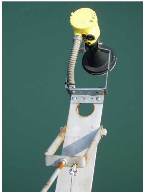
Figure 5. Level measurement by emerged radar. [© EDF DTG]
