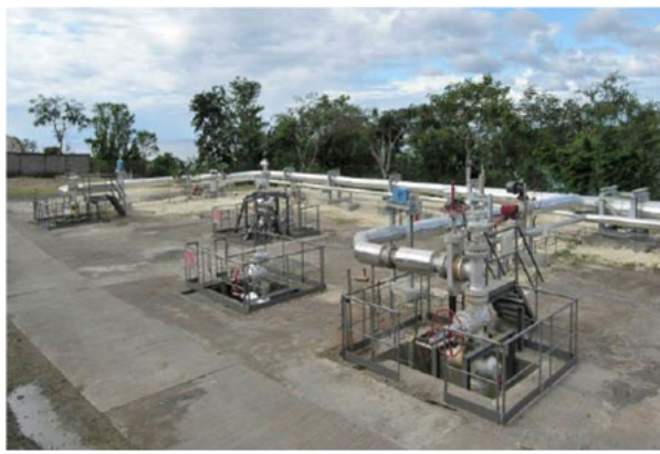
Figure 4. View of the production wellheads of the Bouillante field on the island of Guadeloupe. [Source: photo CFG services]
