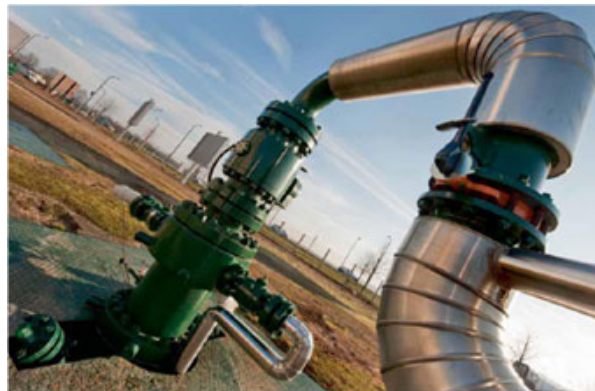
Figure 3. Producing wellhead in the Melun area. Note the thermal insulation required to limit heat loss during flows in the surface piping. [Source: photo ADEME]
