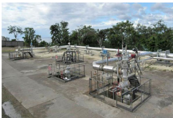
Figure 4. View of the production wellheads of the Bouillante field on the island of Guadeloupe. [Source: photo CFG services]
