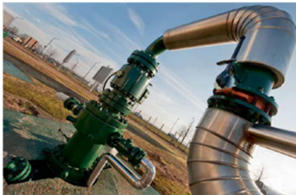
Figure 3. Producing wellhead in the Melun area. Note the thermal insulation required to limit heat loss during flows in the surface piping. [Source: photo ADEME]
