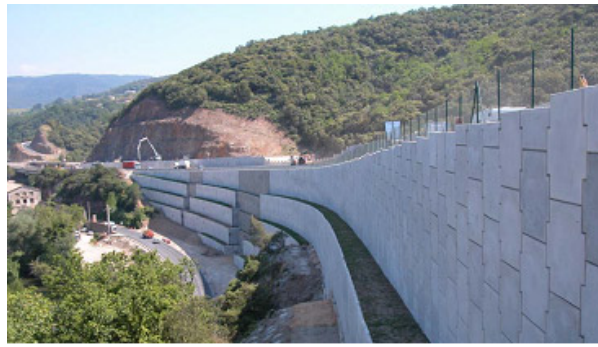
Figure 6. A high retaining wall made of "reinforced earth wall". Each wall level consists of joined reinforced concrete "scales" anchored by friction in the upstream embankment by means of metal rods. The backfill is built as the wall is erected. This technique makes it possible to create aesthetic, stable, sub-vertical and draining walls. [Source: E. Lucas, P. Sery, A. Tigoulet, D. Brancaz, 2008, Les ouvrages récents de grande hauteur en sol renforcé , Compte rendus JNGG 2008 , Nantes]
