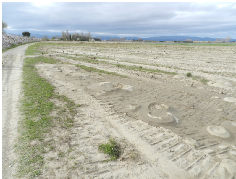
Figure 2: Example of a sand mound resulting from a "sand boil" downstream of a dyke (Agly dyke, March 2013) [Source: © P. Mériaux].
