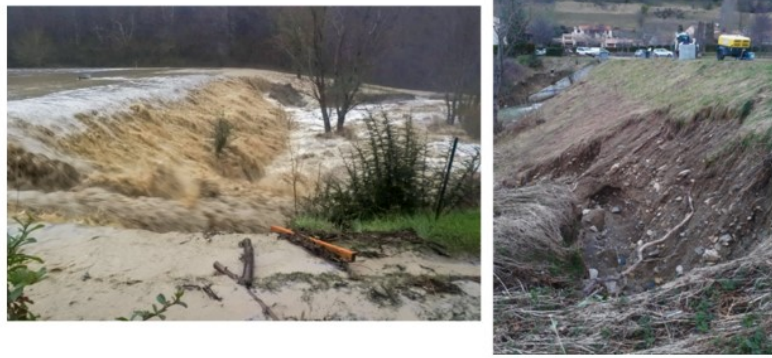
Figure 1: Overflow of the Chalabre dam (Aude department, January 2020) and resulting erosion niche [photos P. Gastineau and A. Wautier].
