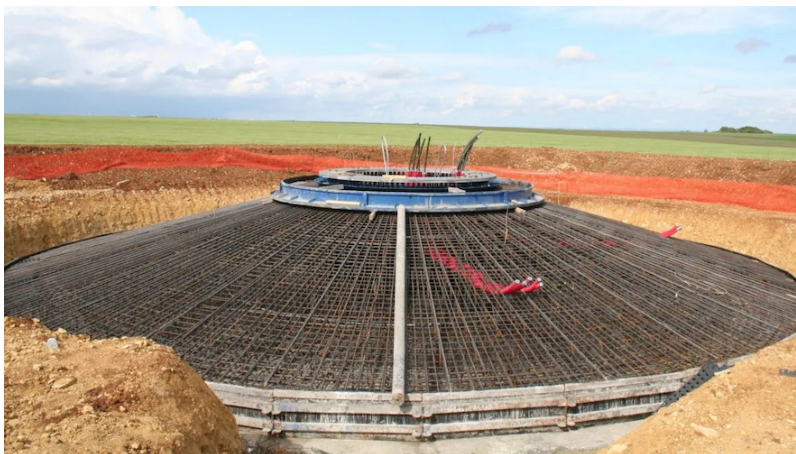
Figure 10. Gravity foundation for multi-MW wind turbine under construction [Source: © Enerfip - Wind turbine foundations: reviewing the basics ]
